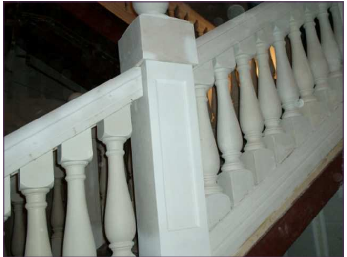
Detailed in the photos shown, is the railing above the post attached to the post cap, while the railing below the post is connected just below the cap.
